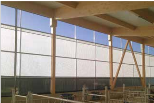
Lubratec roll-up ventilation system for calves, interior view
