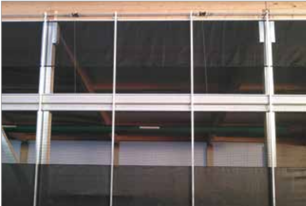
Lubratec roll-up ventilation system for calves, in open position
