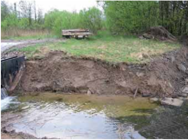
Erosion problems at outlet structure (1)
