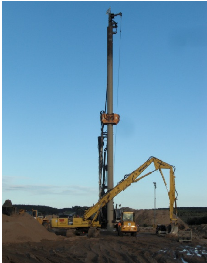
Figure 15. LRB 255 rig with 30 m long displacement pipe on construction site in Poland
