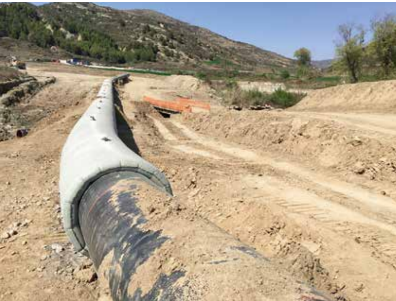
Trans Adriatic Pipeline (TAP) Greece/Albania: protection of pipe against buoyancy, uplift and mechanical actions with Incomat Pipeline Cover.
