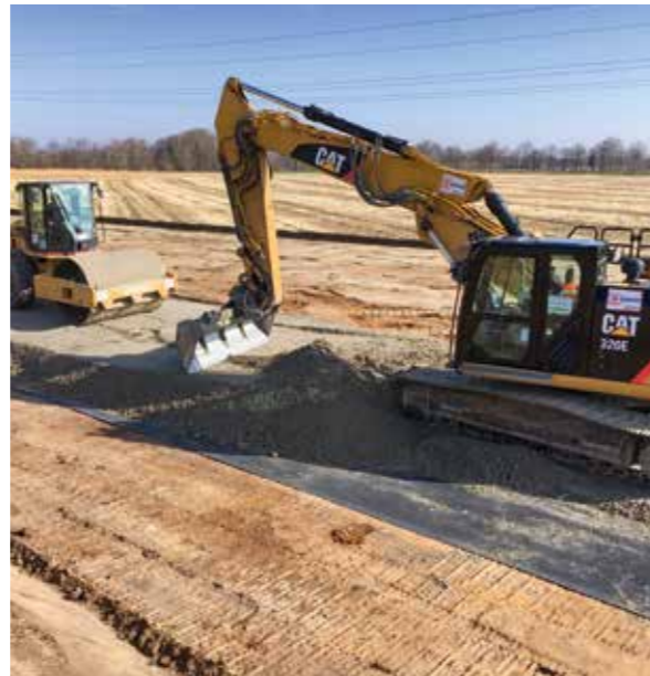
Loop Epe-Legden (LEL) natural gas pipeline, DN 1100 Germany: base reinforcement for continuous haul road alongside pipe trench and storage areas.
