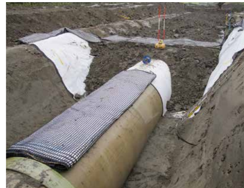
Ballasting of pressure sewage pipe Netherlands: protection against buoyancy and uplift with Basetrac Duo-C geocomposite.
