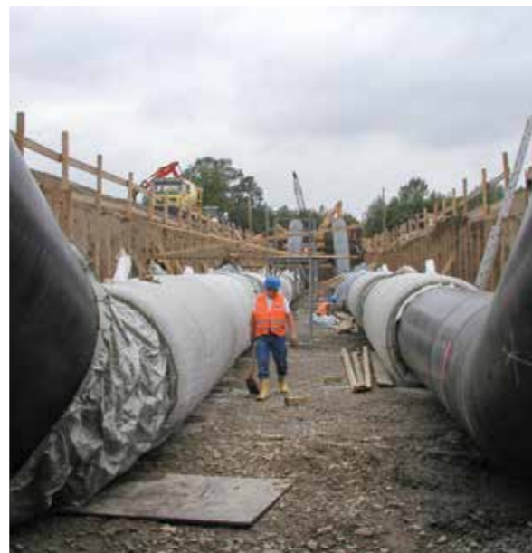
Ruhr inverted siphon, DN 1400 Germany: protection of pipe against buoyancy, uplift and mechanical actions with Incomat Pipeline Cover.
