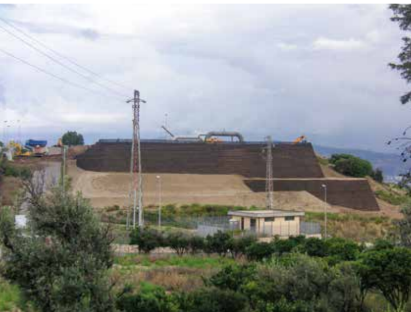
Modernization of gas compressor station Italy: construction of extra-steep, low-settlement and settlement resistant slopes using geosynthetic reinforced soil method.
