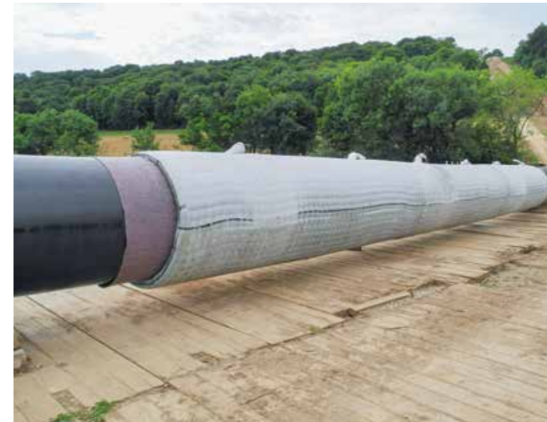
Val de Saône, DN 1200 France: protection of pipe against buoyancy, uplift and mechanical actions with Incomat Pipeline Cover.
