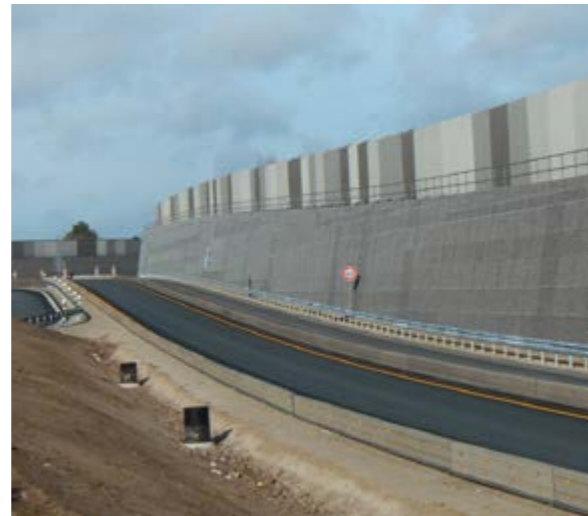
Highly absorbent noise barrier Germany | New highly absorbent noise barrier for six-lane widening of A3/A73 motorways, Fürth-Erlangen – Absorption category A 3 (sound absorption DL_a \geq 8 - 11 dB) – Gabions facing carriageway and vegetation on the other side – Height up to 10 m.
