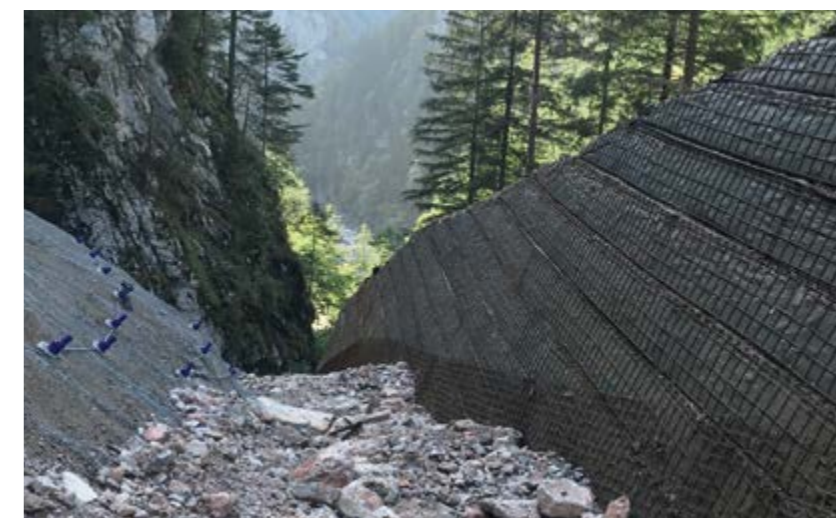
Rockfall protection dam in Gesäuse National Park Austria | Challenging avalanche protection structure in highly inaccessible terrain – Slender dam with 70° longitudinal inclination – Geometry adapted to steep mountain – Built to ONR 2481 regulations – System with integrated lost formwork – 18,000 m² Fortrac MDT (PVA).
