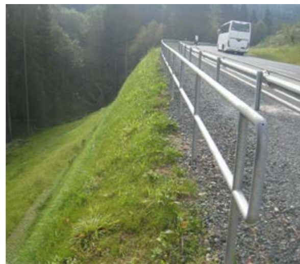
B85 trunk road widening Germany | Trunk road between Lösau and Höferänger directly on geosynthetic-reinforced retaining structure – 11 m tall, 70° inclination, with natural vegetation – System with integrated corrosion-protected formwork.
