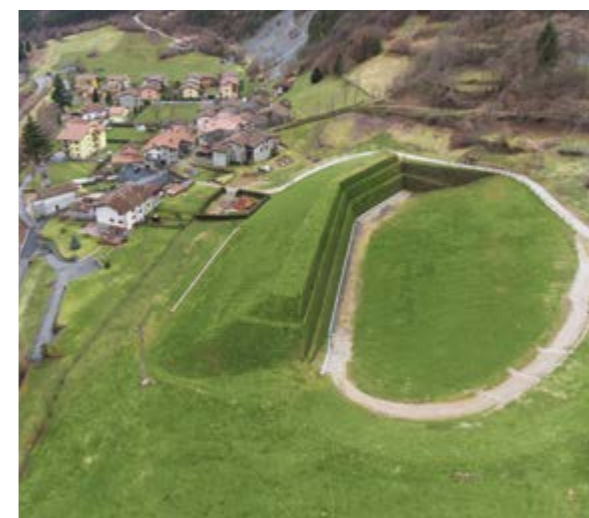
Avalanche protection dam for Ludrigno Italy | Protection of Ludrigno’s population and valley-bottom infrastructure against avalanches – System with integrated lost formwork – Protective structure is approx. 140 m long and 10 m tall.
