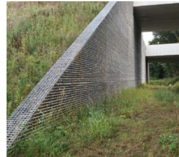
Double bridge abutment for A74 motorway Netherlands | Major project near Venlo, incl. two motorway bridges directly adjacent to each other – Abutment heights 11 m and 9 m – Rapid completion on very soft subsoil – Phased installation after advance surcharging – Tie rod system.
