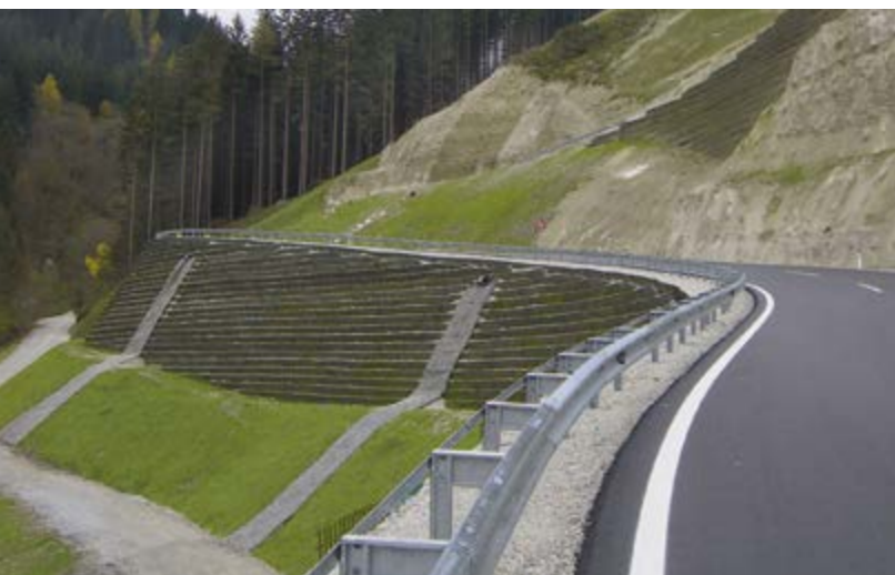
New road – Triebener Straße B114 Austria | New-build road offering reliable long-term performance on active creep-prone slope – Made possible by high ductility of GRS – Grid mesh size adapted to local fill material – System with integrated lost formwork – Retaining structure up to 28 m tall.
