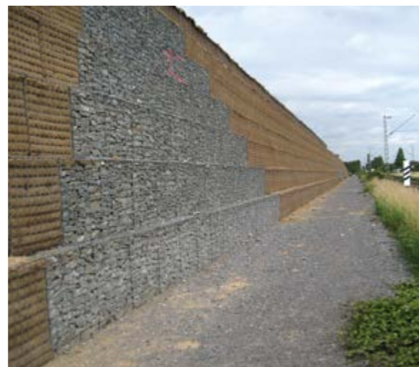
Noise barrier for residential estate in Neuss Germany | Development area by railway and regional road – Combination of full-gabion wall facing track and natural slope facing new housing – Gabions filled with stones, soil and vegetation – 10 m tall with 68° inclination on track side.
