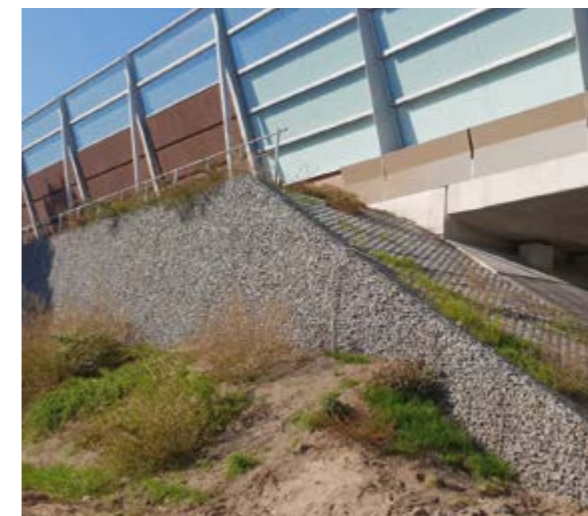
Motorway widening within existing footprint Netherlands | Six-lane widening of (A1/A27) motorway section near Utrecht – Natural sloping motorway embankment rebuilt as steep slope with Fortrac Gabion tie rod system – Erection of top noise barrier made possible by integration of concrete pile supports in system.
