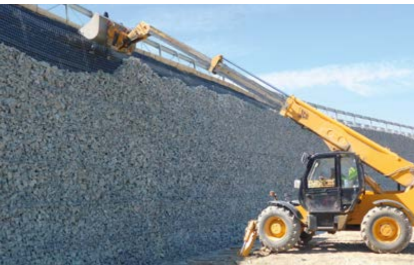
Approach ramp for new bypass motorway Romania | 200 m long, 11 m tall approach ramp (A4 motorway, Constanța-Poiana) – Tie rod system – Special steel mesh aperture size – Rapid progress on site e.g. through simplified filling operation with easy-to-use plant and (140 mm dia.) natural fill material.
