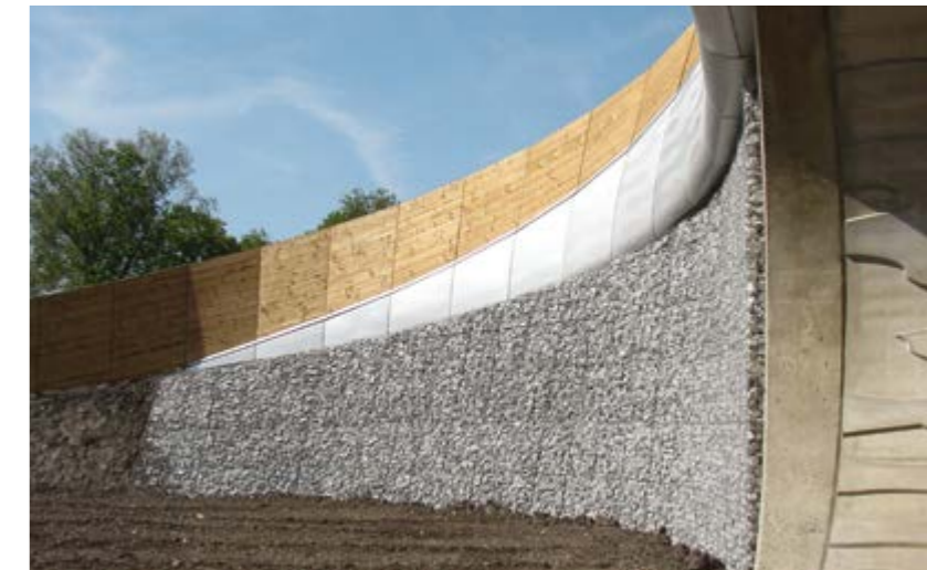
Modern wildlife bridge over A2 motorway Netherlands | Vegetated wildlife bridge over A2 motorway – Curved approach ramp topped by modern architectural feature – Fortrac-reinforced soil system applied in conjunction with half-gabion facing – Height approx. 8 m.
