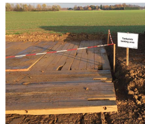
Temporary construction site gas stations Germany | A temporary refueling area for construction machinery was created for a greenfield construction project. The use of Tektoseal Active AS protects the substrate from fuel spills. The wooden planks above the filter mat ensure trafficability and protection of the mat e.g. against UV radiation and mechanical impacts.
