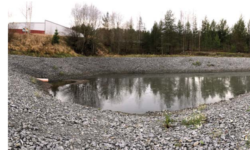
Mine water treatment Finland | Mine drainage containing metal can also be treated in basins next to pits and heaps. For mine water treatment in a closed nickel mine, two filter basins were lined with Tektoseal Active HM.
